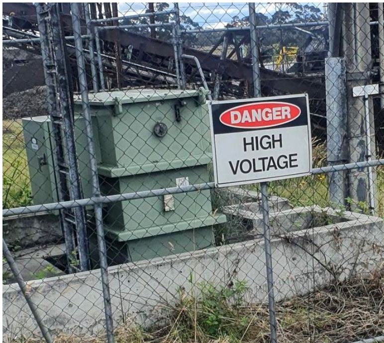
Pad Mounted Transformer at Pole 1
